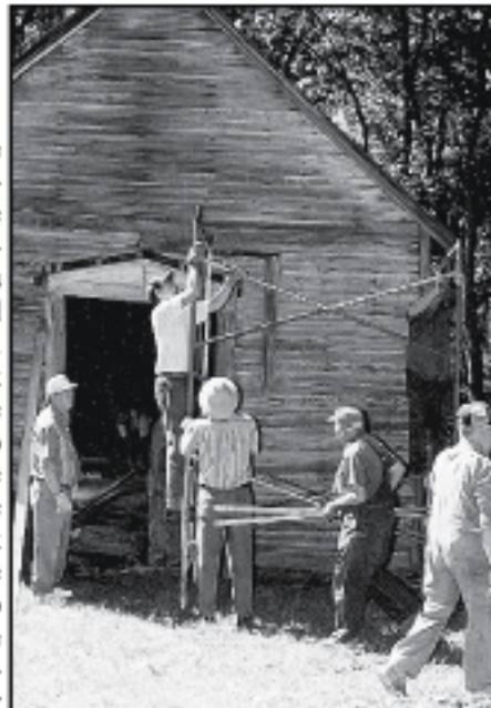
Between the Rivers volunteers work on the facade of the old St. Stephen Church in this July, 2000 photo. Paducah Sun file photo
