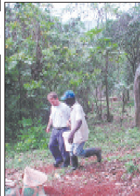
Fr. Ken and Myrie - carrying water for mixing concrete for the Food for the Poor Home in progress (this will be Myrie's home)
