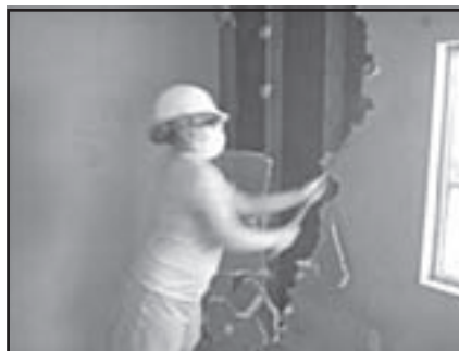
Lyndsey Bernard uses a bar to remove molded drywall from Ms. Evelina's house.
